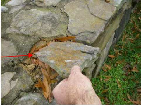
Samples: Missing stones Loose stones
